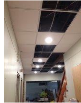
Ceiling and LED Lighting
